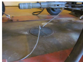
Example of a floor drain illicitly connected to a storm drain
